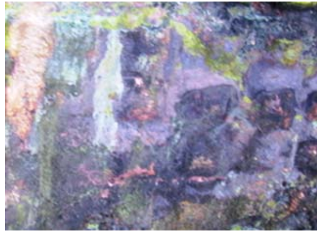
Figure 7. Severely corroded, unprotected copper block. Black copper sulphide pervasive. Increasing evidence of green copper hydroxychloride in close proximity to copper
