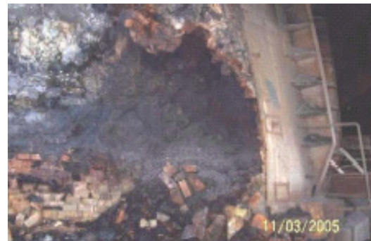
Figure 8: Right side Cavity after brick movement due to distortion
