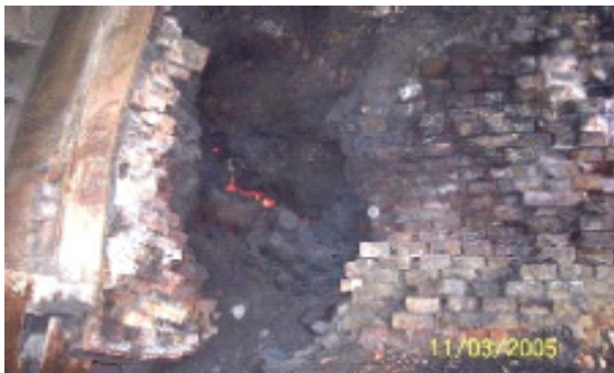
Figure 7: Left side Cavity after brick movement due to distortion
