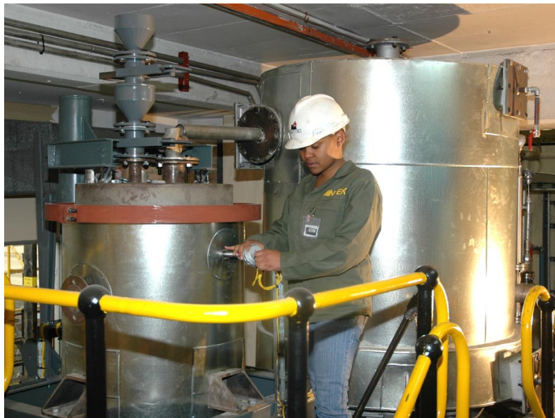
Figure 3: Chlorinator and iron chloride condenser at Mintek pilot plant
