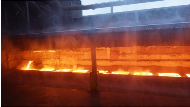
Figure 8: Permanently mounted water sprays along the casting bed roof. No fume is escaping from under the roof.
