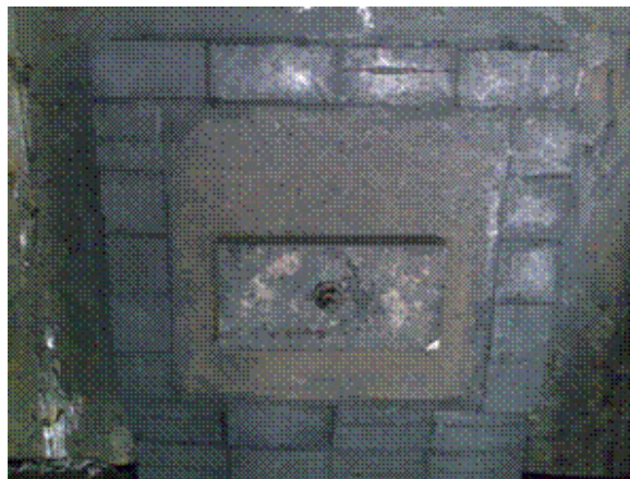
Figure 9: Tap block and surrounding bricks inside steel flange as see from outside of furnace
