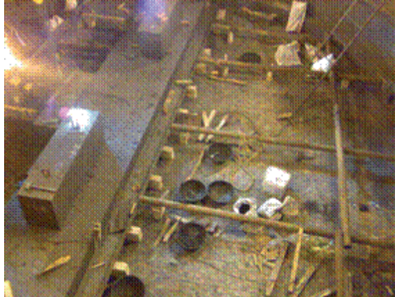
Figure 7: GradeD™ carbon block in hearth showing proper jacking by means of jacks and wooden poles
